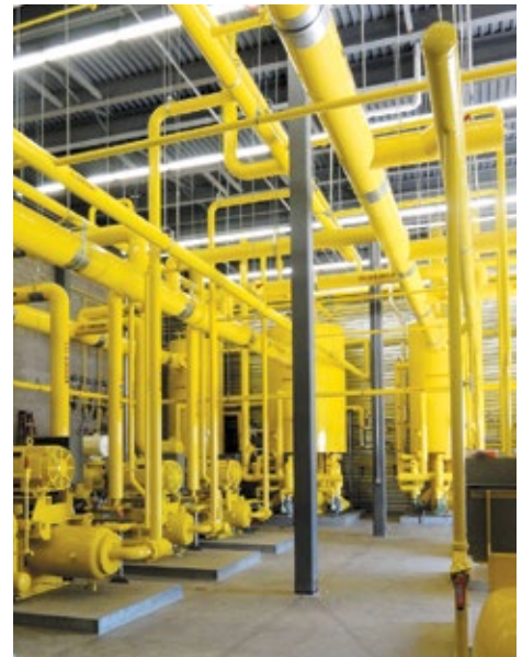
■ The rack steel in this 902,000-square-foot distribution center weighs 8,027,899 pounds or 4,013 tons. The ammonia refrigeration piping is 29,244 feet long or 5.54 miles.
